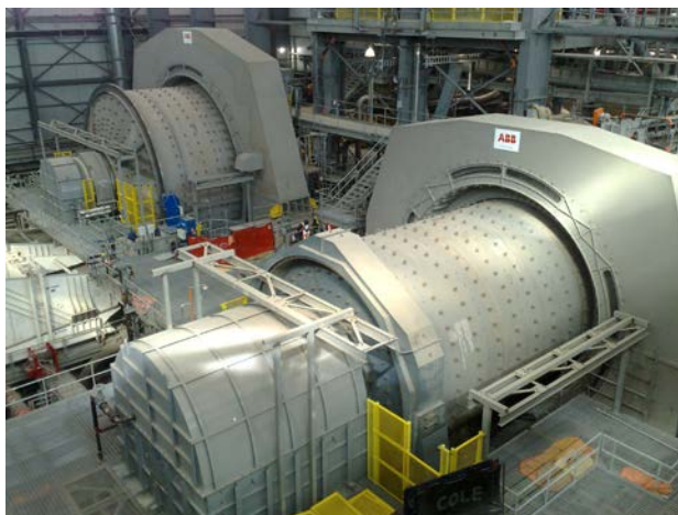
ABB GMD at Climax Molybdenum Mine
